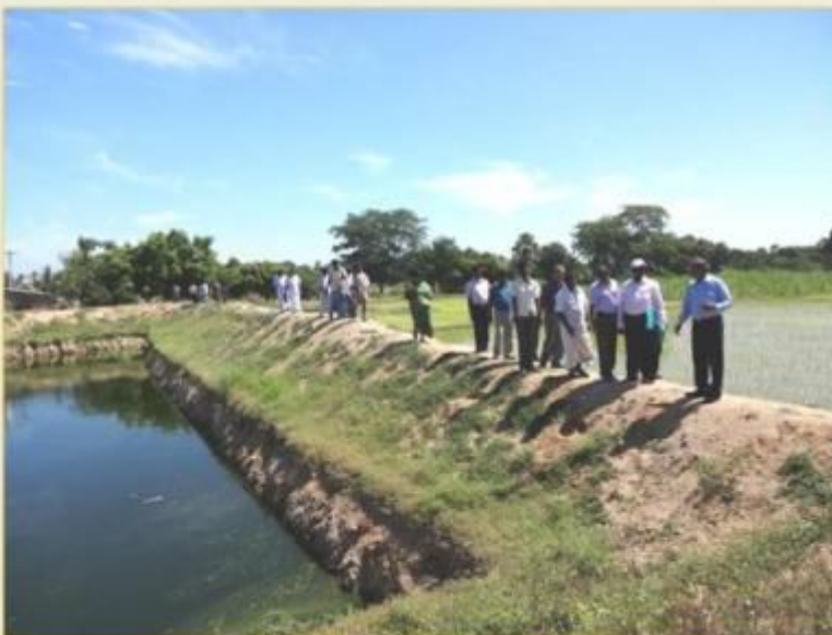
Rainwater harvesting structure in NICRA Village
